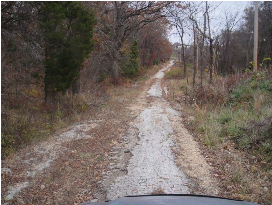
View to the east along Golf Road. Note significant deterioration of roadway, absence of curbs, gutters, shoulder, sidewalk. Also limited visibility in certain locations.
