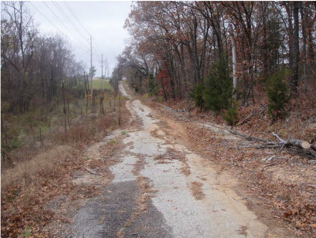
Golf Road west end, photo showing significant drainage ditch along side of road.
