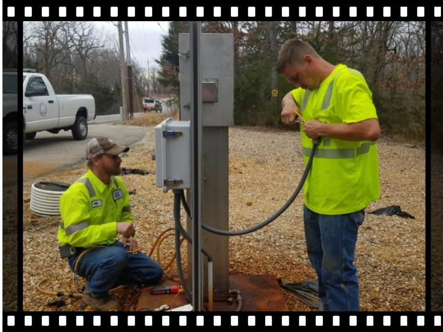
Chad Stark and Dustin Walker (Sewer Department) handling repairs to the odor control facility on Dude Ranch Rd.
